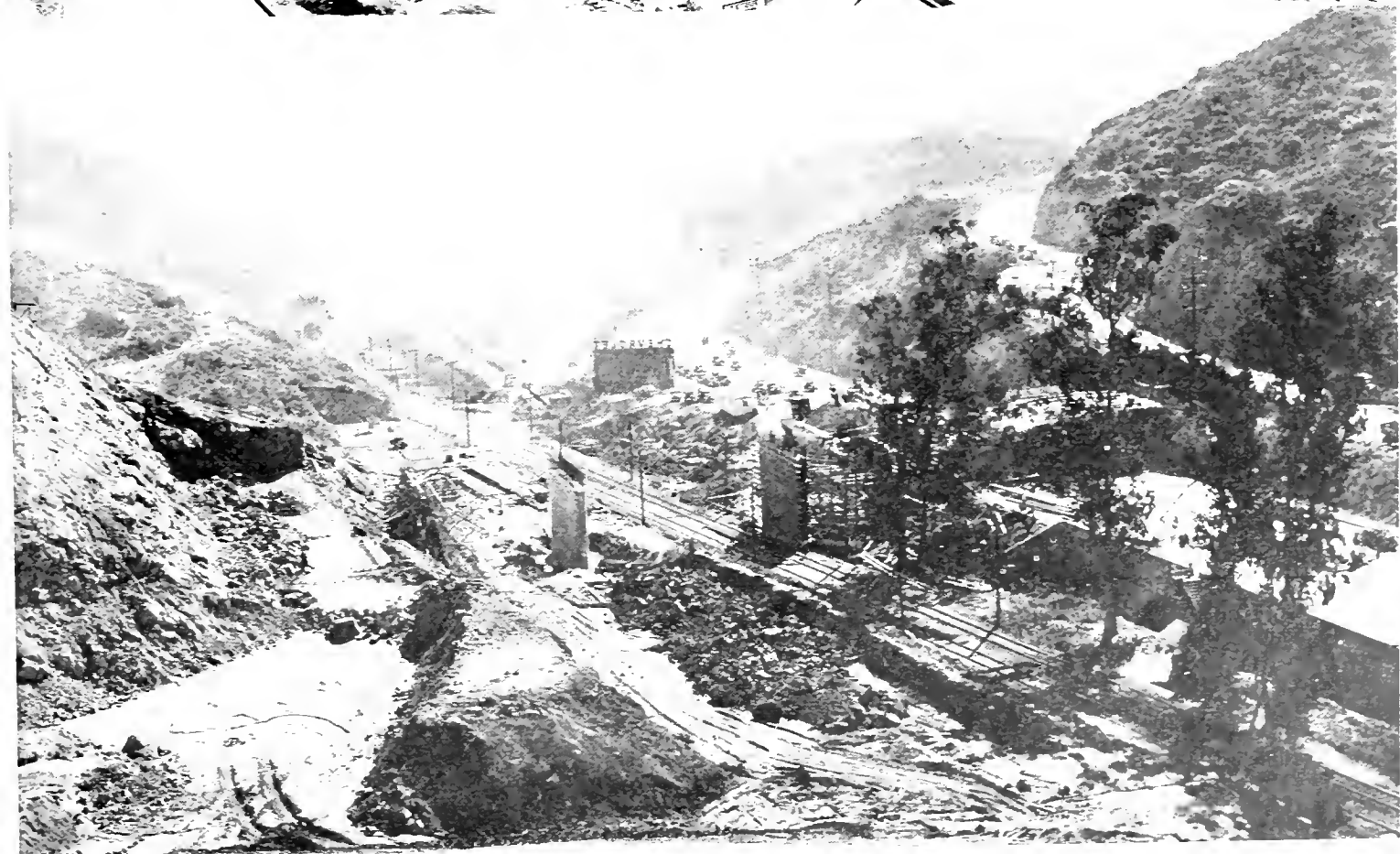
At top—General view of new Canuenga Pass Freeway section looking south. Mulholland Drive overpass structure in foreground spans the old pass road retained as a service road on the right, the two 4-lane freeway roads, depressed railroad tracks and service road on the left. Lower picture shows scene during construction when railroad tracks were moved to a center position between freeway lanes.
